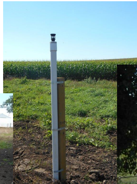
Irrigation Riser and Example of Established Irrigation Area with Sprinklers Running
